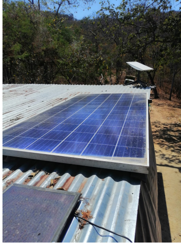
Figura 3.9: Panel solar instalado
