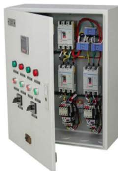
Figura 13. Caja de panel de control [29]
