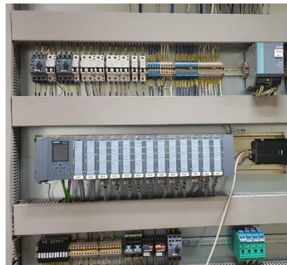
Figura 23. - Tablero de Control (Parte Interna). (TESSIS SUPPORT AUTOMATION & CONTROL, 2020)
