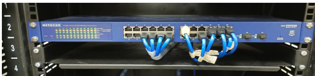
Figura 17. Smart Switch ethernet
