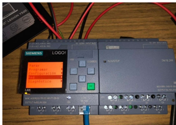
Figura 16. Controlador PLC Logo 12/24RCE
