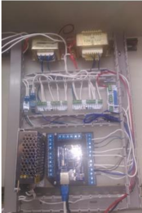
Figura 29 Panel de control
