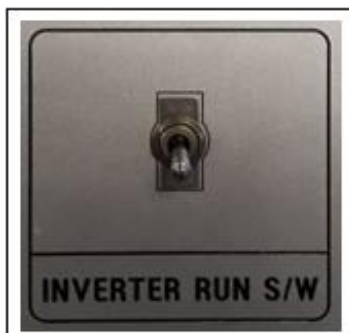
Figura 24 control de inversor
