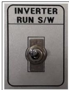
Figura 46. Control de inverter
