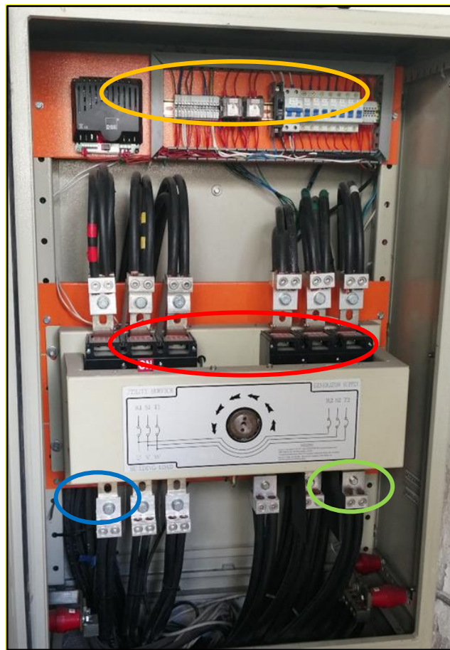
Figura 13. Tablero principal “ATS”.
