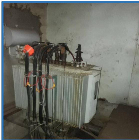
FIGURA 30: TRANSFORMADOR 13.8 KV / 380 V.
