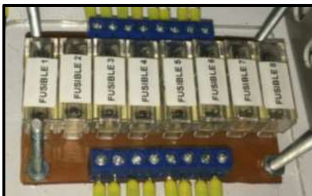
FIGURA 19: TARJETA PORTA FUSIBLES.
