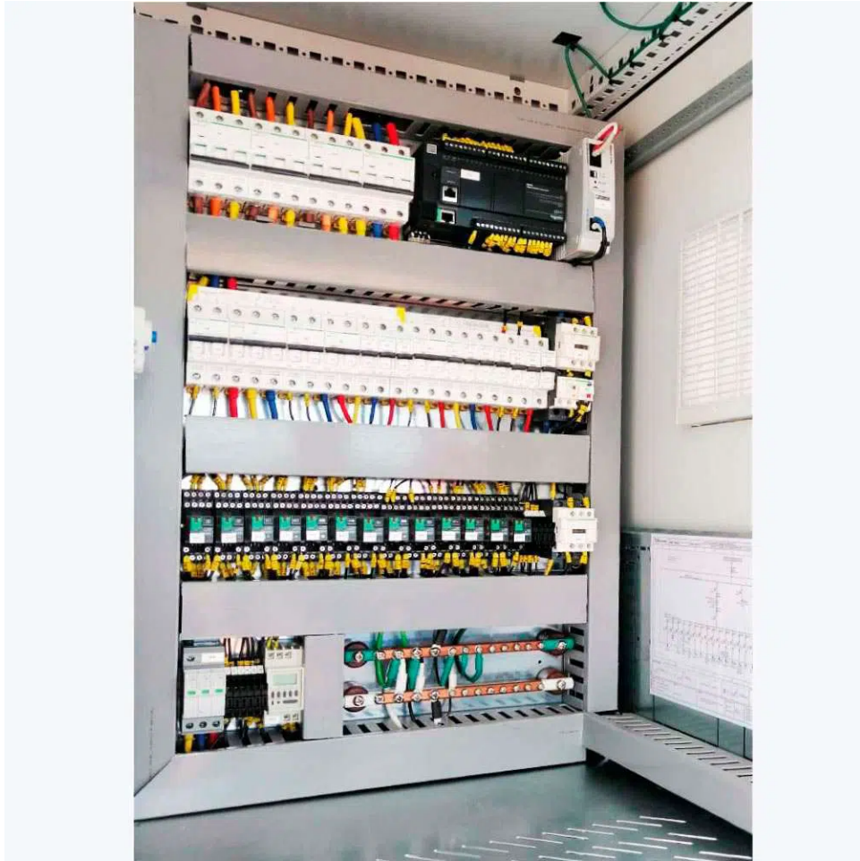
Figura 6. TABLERO DE CONTROL
